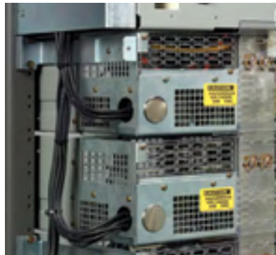
Bottom AC Wireway Input (cover removed)
