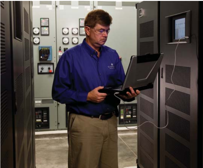
The Liebert NXL UPS from Emerson Network Power provides reliable power protection and advanced technology for the global data center's high-power applications.
