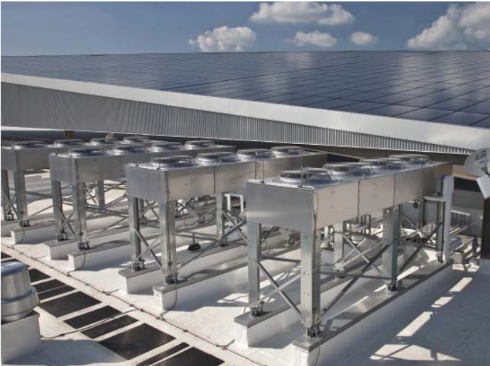
By placing the chillers on the roof, Emerson's data center planners not only conserved real estate, they eliminated more than two miles of copper pipe.
