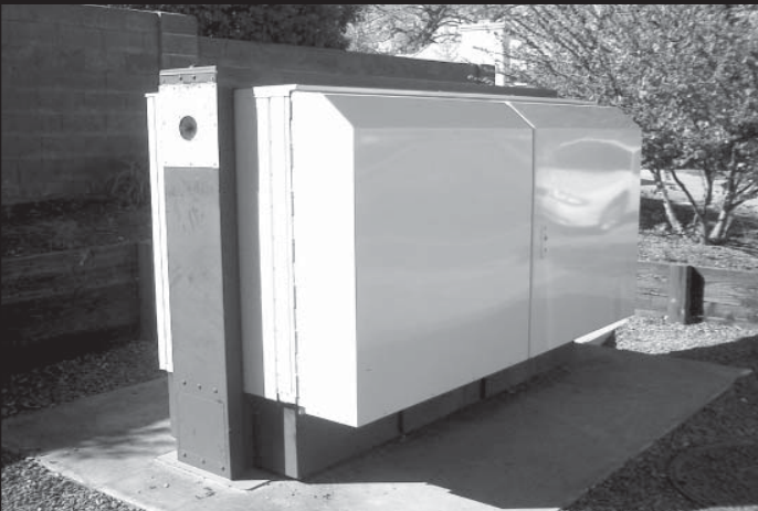
Figure 7: Acoustic hoods redirect sound, but may compromise GR-487 compliance.
