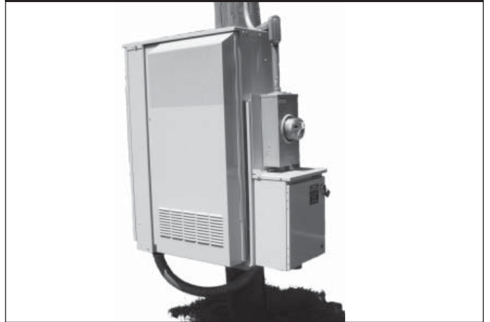
Figure 6: Orienting door-mounted heat exchanger toward street directs sound away from neighbors.
