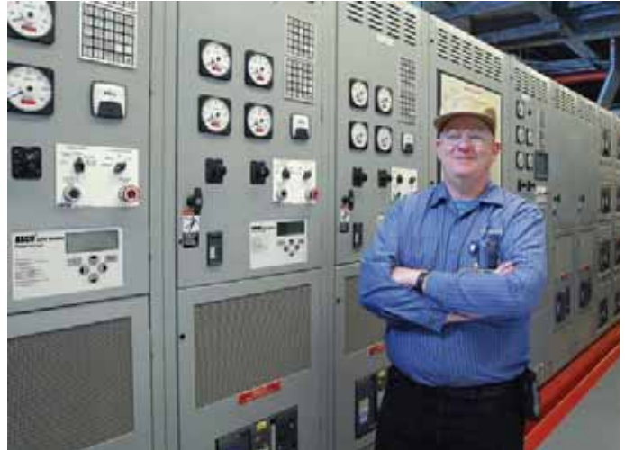
Kevin Deitsch, electrician at St. Joseph's, monitors performance of the hospital's emergency power systems via ASCO PowerQuest®.
