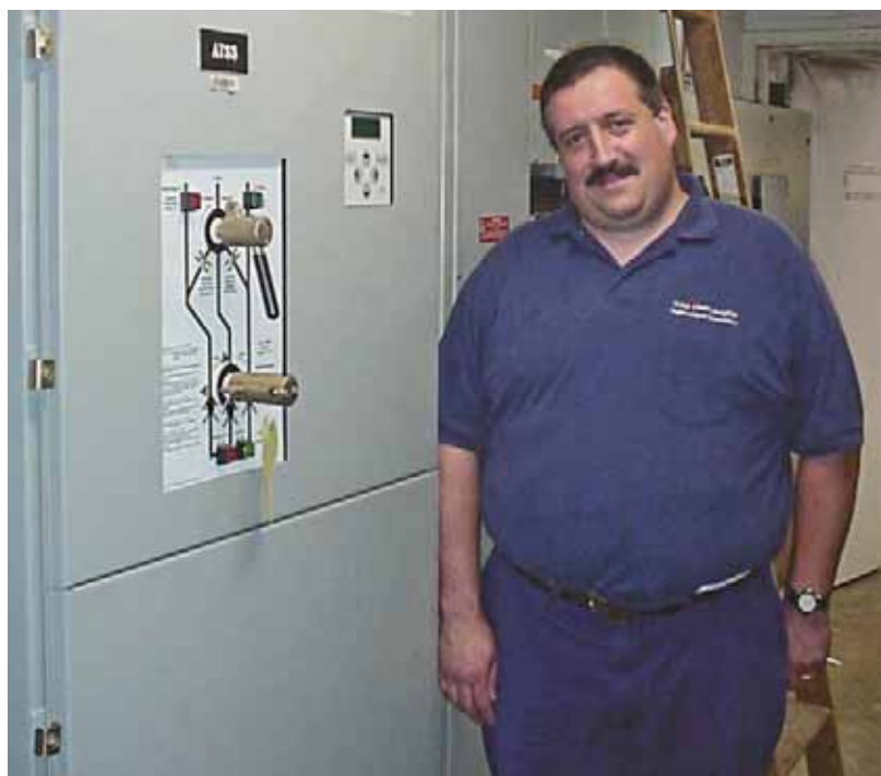
Cliff Blewett, electrician at Saint Clare's Hospital, was part of a brain trust of hospital engineering staff, an electrical contractor and ASCO that quickly replaced a competitor's failed power transfer switch. He is standing next to an ASCO Bypass-Isolation Power Transfer Switch.
